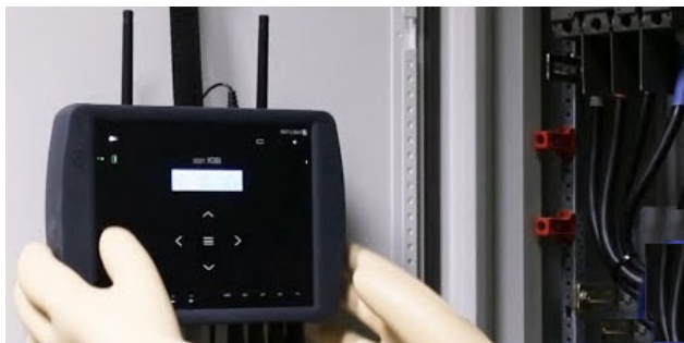
Fig. 3. Installation of MYeBOX 1500 in a distribution panel.
